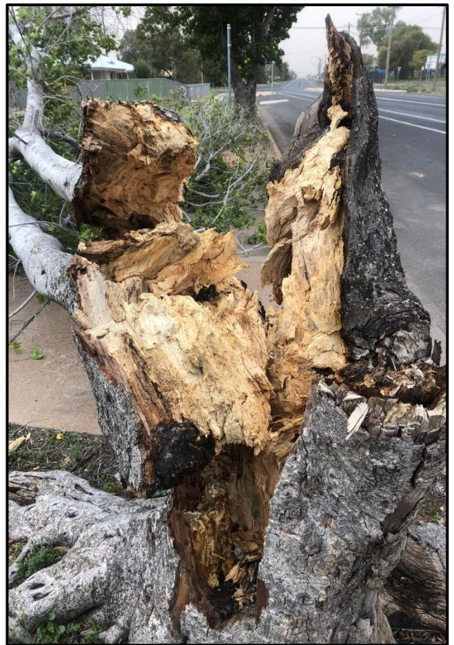
Photo of the decaying timber
