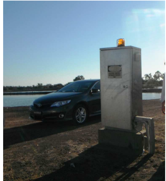
Figure 4.8 – Effluent recirculation pump switchgear
