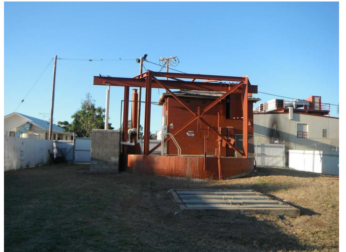
Photo 4.2 – Mertin St SPS (SPS 2)
