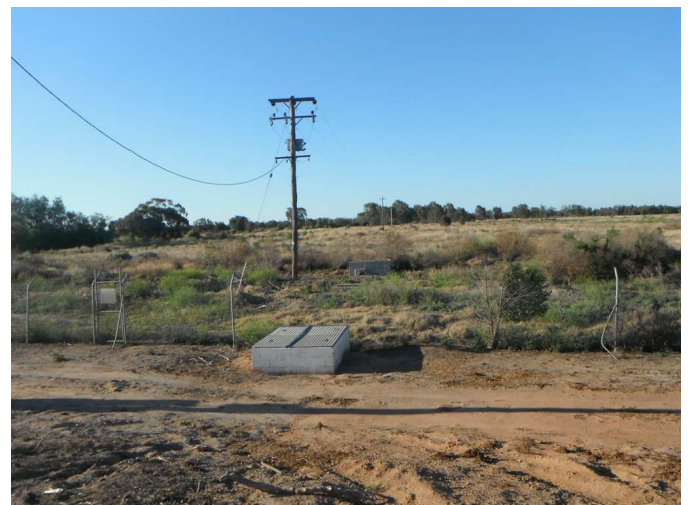
Figure 4.9 – Effluent discharge pit and overflow pit (in background)
