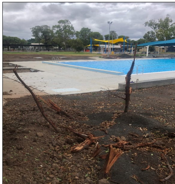
Roots from excavation in close proximity to main stormwater drain.
