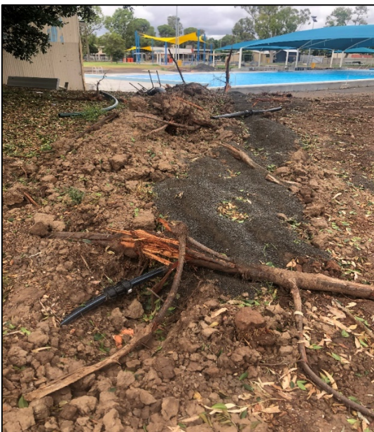
Roots from excavation work (entwined around water service)
