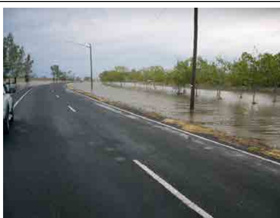
Plate 61 – Floodwater at point of surcharging the Mitchell Highway to the east of the intersection of Bloxham Street and Meadows Road. (Source: Council)
