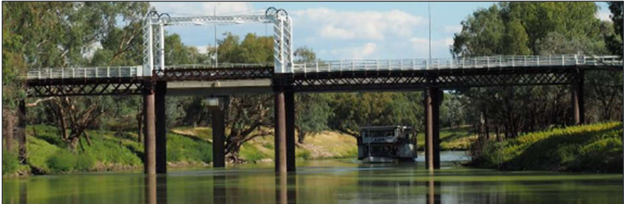
Figure 1-3: General view of the North Bourke Bridge, looking south. Source: Focus Bridge Engineering (FBE), 2024
