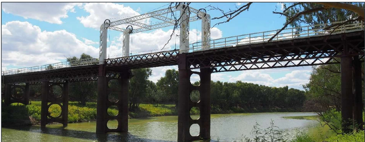
Figure 1-4: View of North Bourke Bridge iron lift and lattice girder spans, looking north. Source: FBE, 2024
