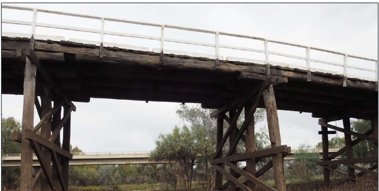
Figure 1-5: View of North Bourke Bridge timber approach girder span, looking south. Source: FBE, 2024
